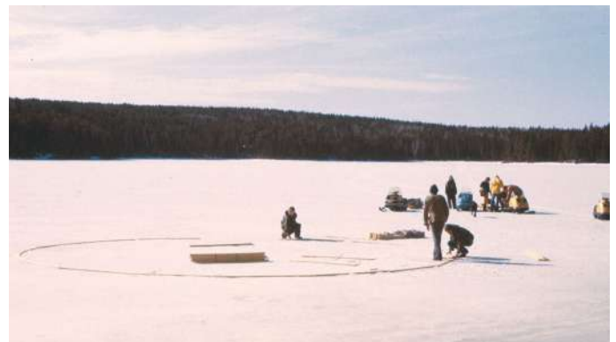
A camp crew has arrived to begin the two-day task of assembling and constructing the flotation frames for the 10 metre mesocosms to be installed in Lake 223 for the acidification pilot studies. (6 April 1976 at Lake 223)
