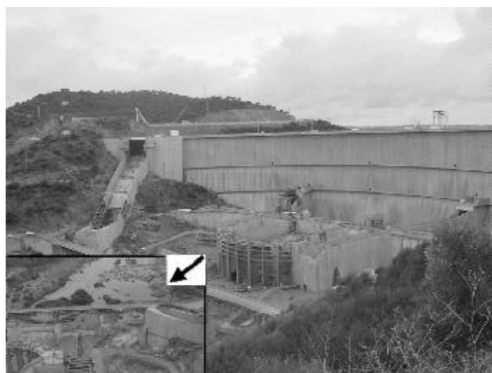
Figure 3 – The Alqueva Dam and downstream river flow (section with arrow), September 2002. Photos are courtesy of Meryem Beklioglu.
